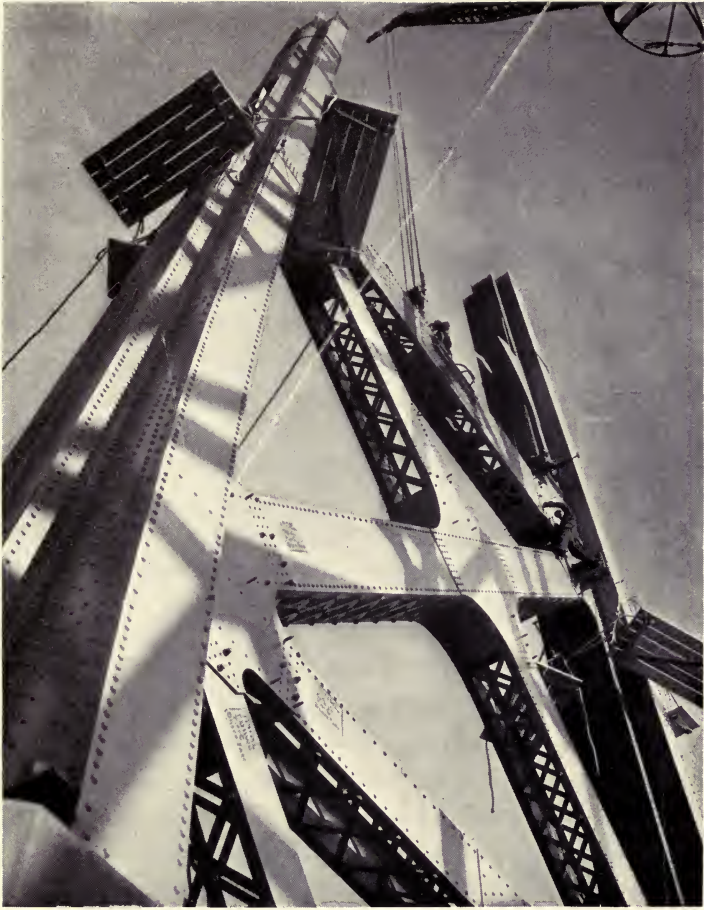
A suspension tower for the Davenport, Iowa, bridge nears completion. This project is being constructed with a loan and grant allotment of $1,527,400 from the Public Works Administration. It is estimated that it will provide 3,600 man-months of employment.
