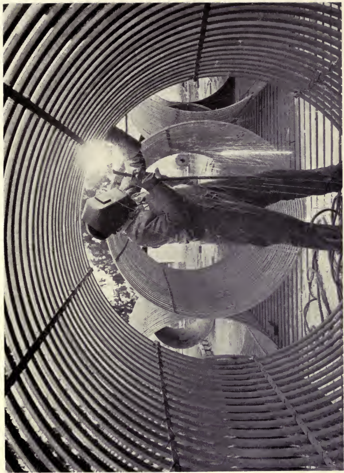
Welding joints in the reinforcing steel used in the concrete pipe for the water supply line from the Hetch-Hetchy dam in the Yosemite Valley. Besides providing an adequate water supply system for the next sixty or seventy-five years, this PWA project will provide 26,700 man-months of direct employment.
