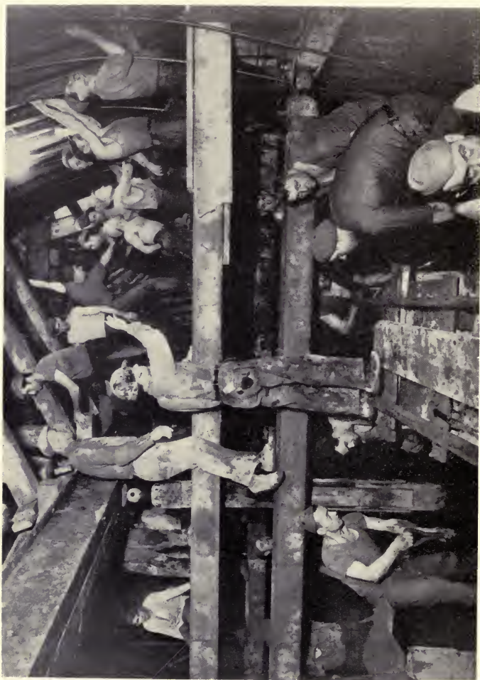
This is not a mural, but a picture of men working on a typical sewer tunnel under a busy Chicago thoroughfare. This immense sewage disposal project, the largest of its kind in the world, is financed with an allotment of $42,000,000 from the Public Works Administration.
