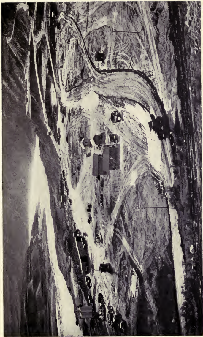
Excavating the west bank of the Columbia River for the Grand Coulee dam and power project being constructed by the Bureau of Reclamation with an allotment of $15,000,000 from the Public Works Administration. This project will cost about $63,000,000 and will produce 2,200,000,000 kilowatt-hours of firm energy; 42,300 man-months of direct employment will be provided.
